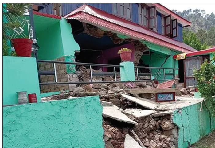
Figure 21 : Houses damaged in Ramban/ Source: Mint _ 26/04/2024 (Media)
