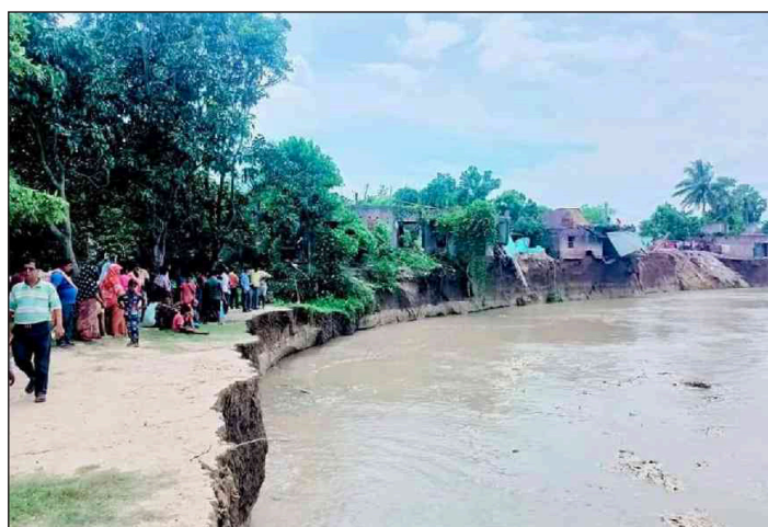
Figure 33 : Eroded banks of the Ganga at Shibpur village in Murshidabad | Source: Media
