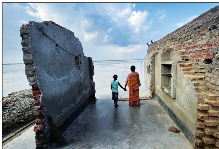
Figure 22 : Damaged House in Murshidabad | Source: Frontline _ 18/08/2024 (media)
