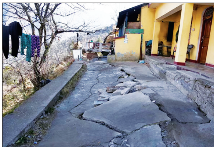
Figure 32 : Joshimath Land Sinking Areas/ Source: Media_13-01-2023
