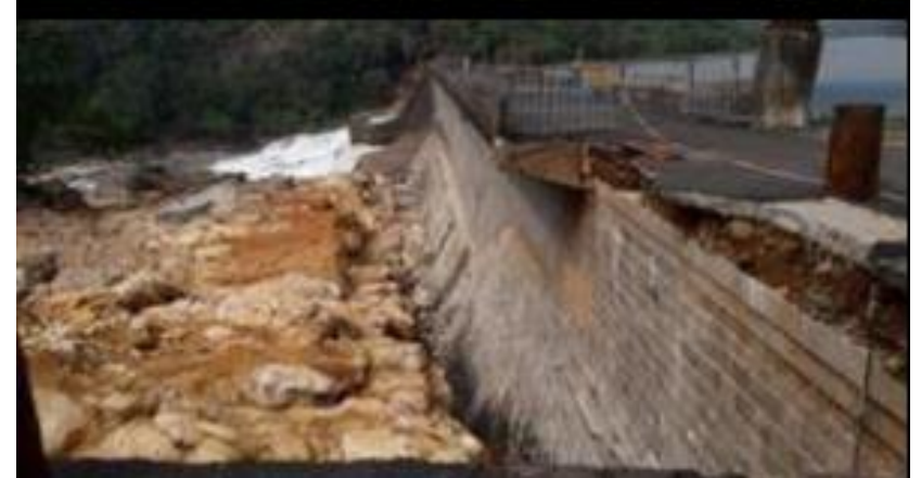
Poringalkuthu Dam (India) before, during and after the overflow.
