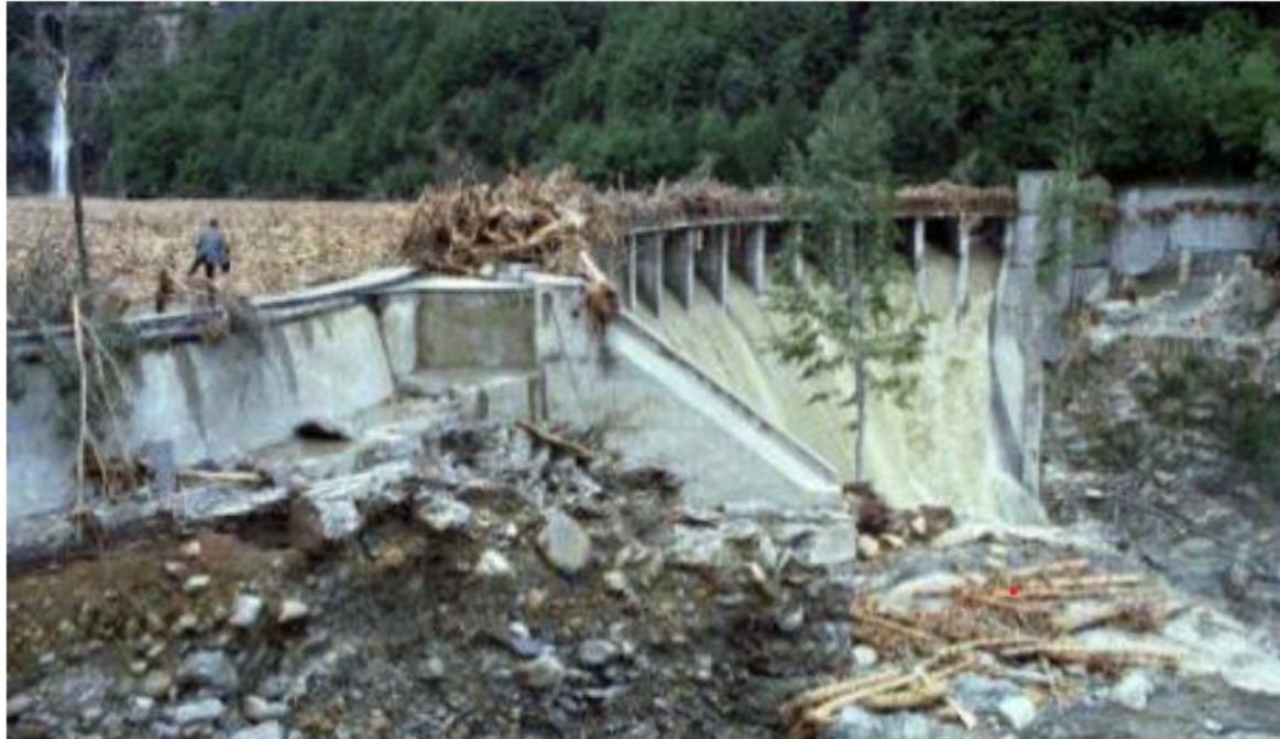
Palagnedra dam, Switzerland – Floating debris
