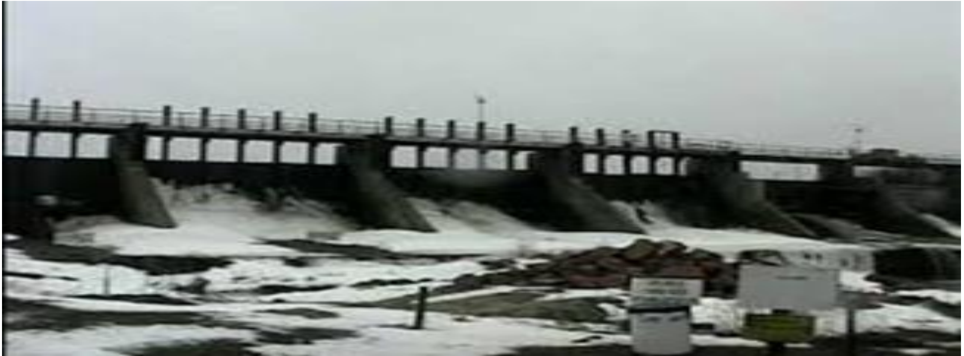
ICE ACCUMULATION IN SPILLWAY
